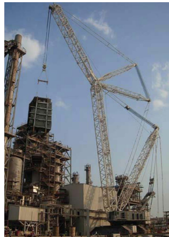
Installation of a 120 te boiler (above) using a Demag CC8800 in Qatar.
