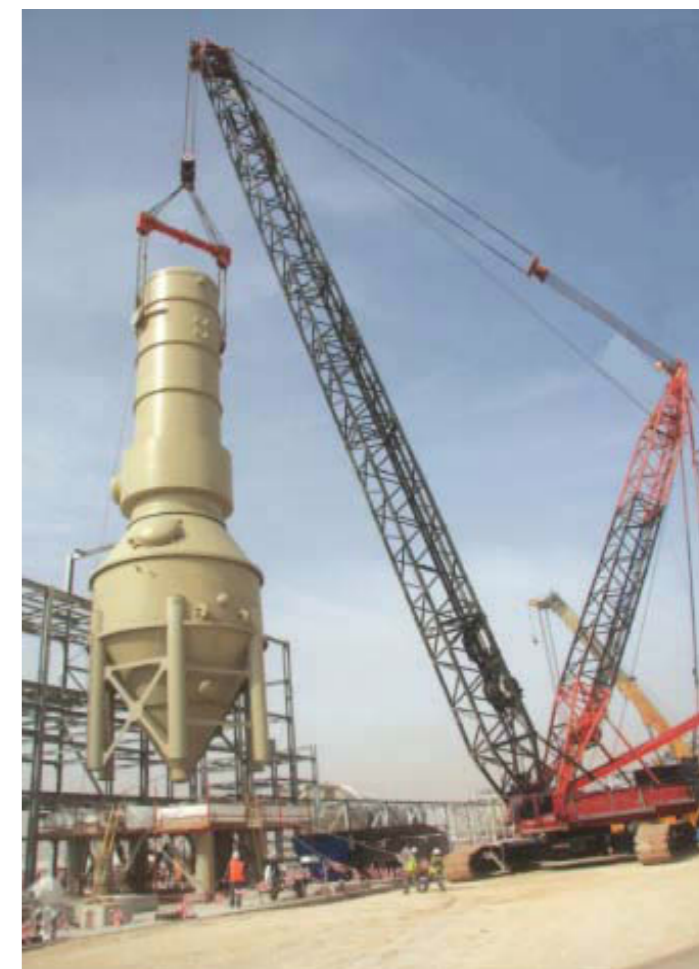
Installation of a 240 te brine evaporator (above) using a Demag CC 2500 as main crane and Demag CC1800 as tailing crane in Qatar.
